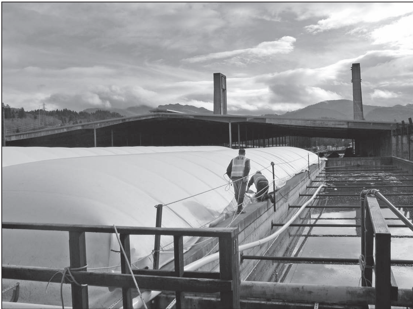
Workers at the Tillamook Biogas Facility in Tillamook, Oregon, check the Hooley Digester, which processes dairy manure and turns it into electricity and compost fiber. Photo by Dorene White, Tillamook PUD.
