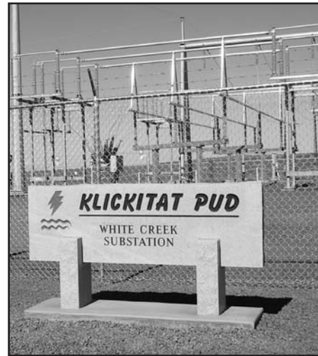
KPUD's new White Creek Substation.
